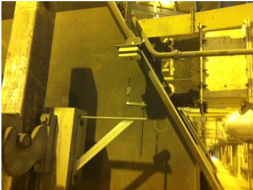
Figure 2. Potentiometer installed on anode beam on cell B114.
